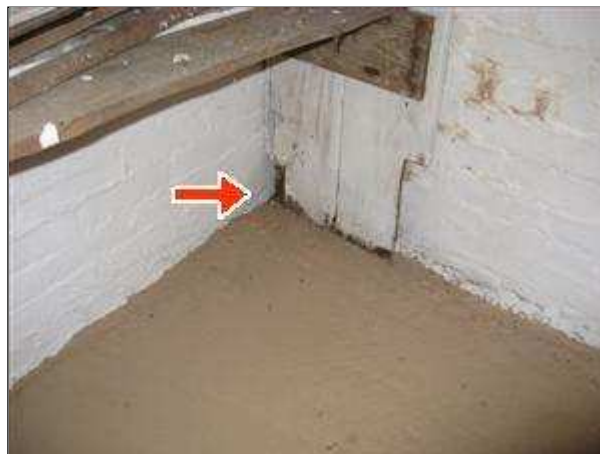
4.0 Picture 2 basement wall
