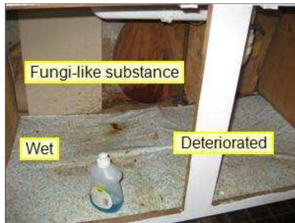
3.4 Picture 1 under kitchen sink
