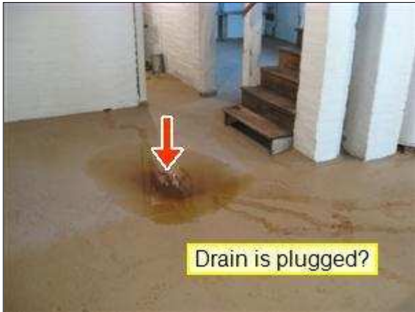
5.0 Picture 4 basement floor drain
